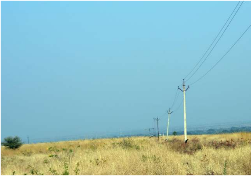
11 kV powerline passing through core area of the GIB Sanctuary from Akolekati to Madri
