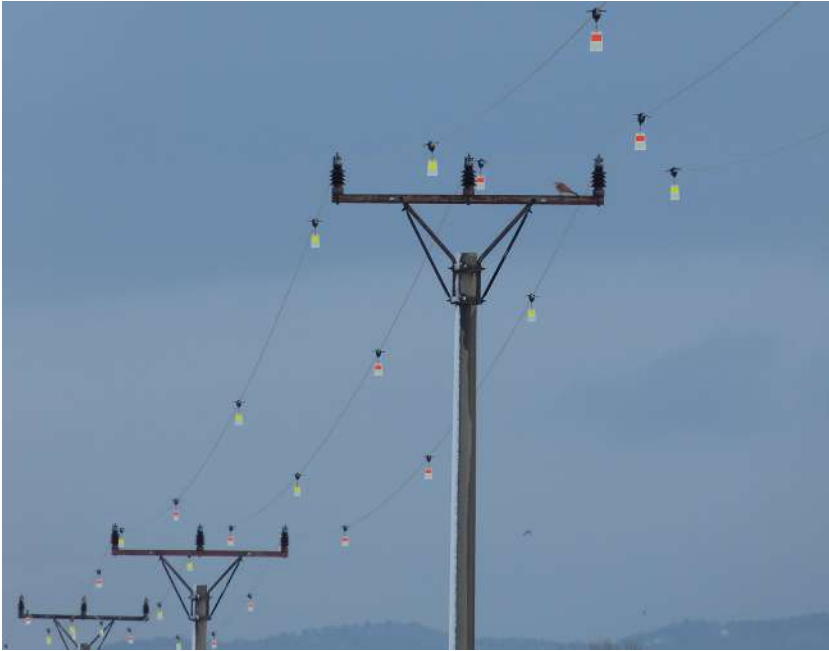
UV-stabilized FireFly Bird Flight Diverters are highly reflective during the day, and continue to glow for up to 10 to 12 hours post sunset
