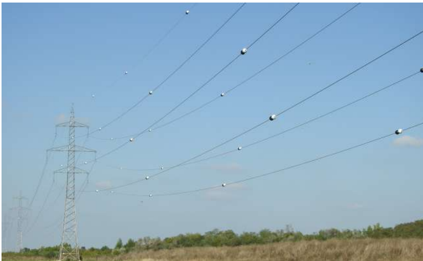
Double black and white aviation marker balls employed for 220 kV power lines, with one marker placed every 30–35 meters along the earth wire and conductor
