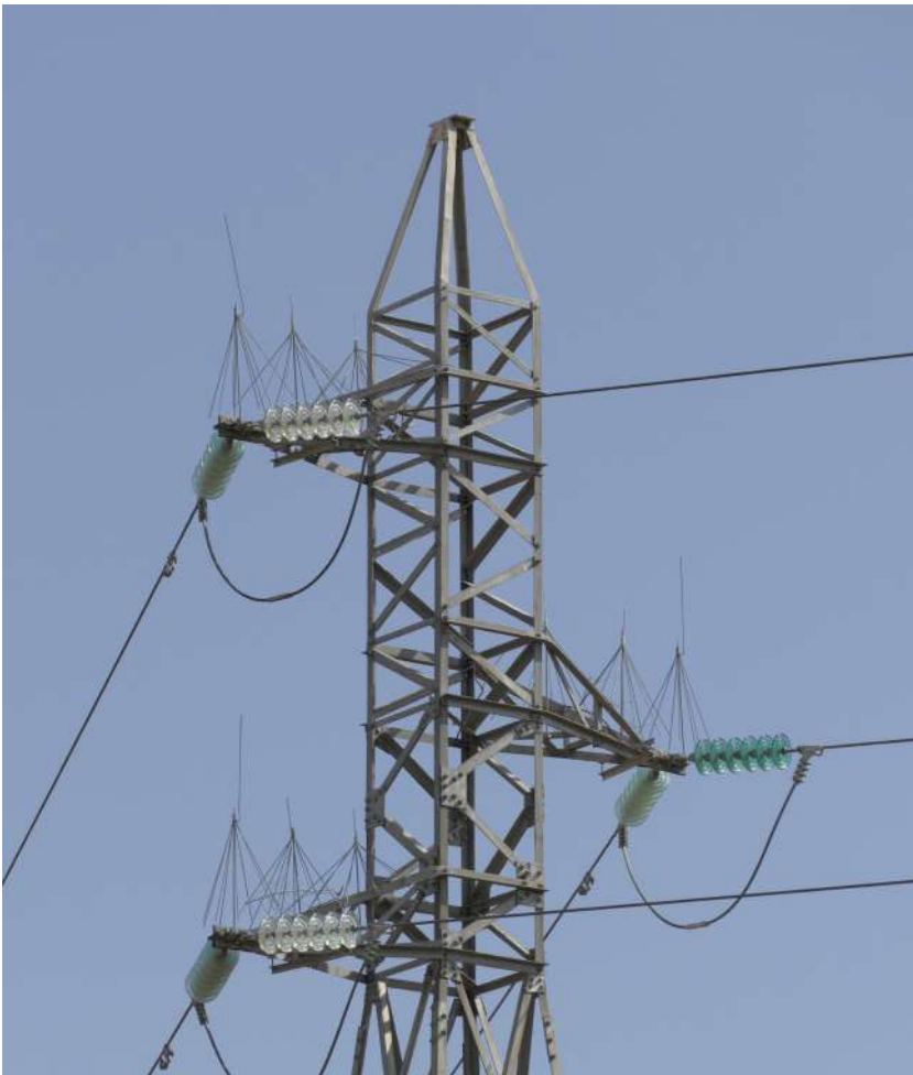
(Top): Various anti-perching deterrents discourage birds from perching on hazardous surfaces or structures – Sturdy metal plates; (Bottom): Fixed metal anti-bird spikes with an umbrella configuration
