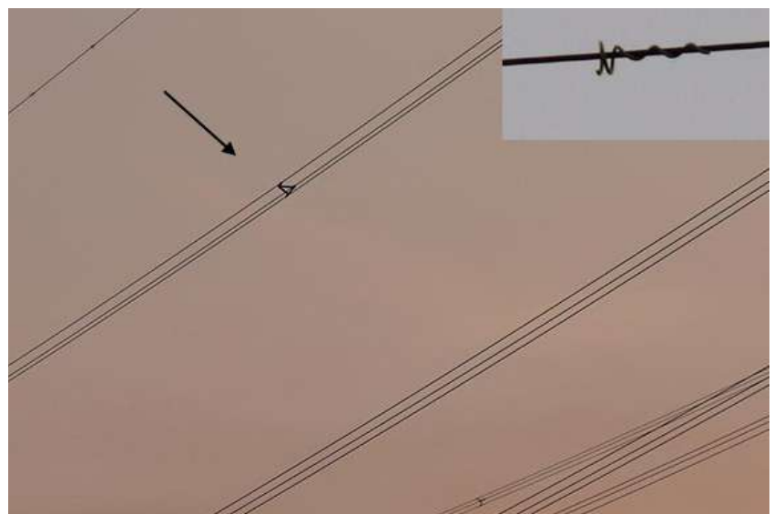
Visibility of wires is enhanced by bundling of a high-voltage transmission line at 380 kV featuring spacers (indicated by an arrow) designed to maintain separation between individual energized phase conductors within each bundle
