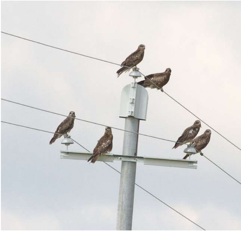
The insulation of crossarms is pivotal for safety enhancements in certain setups
