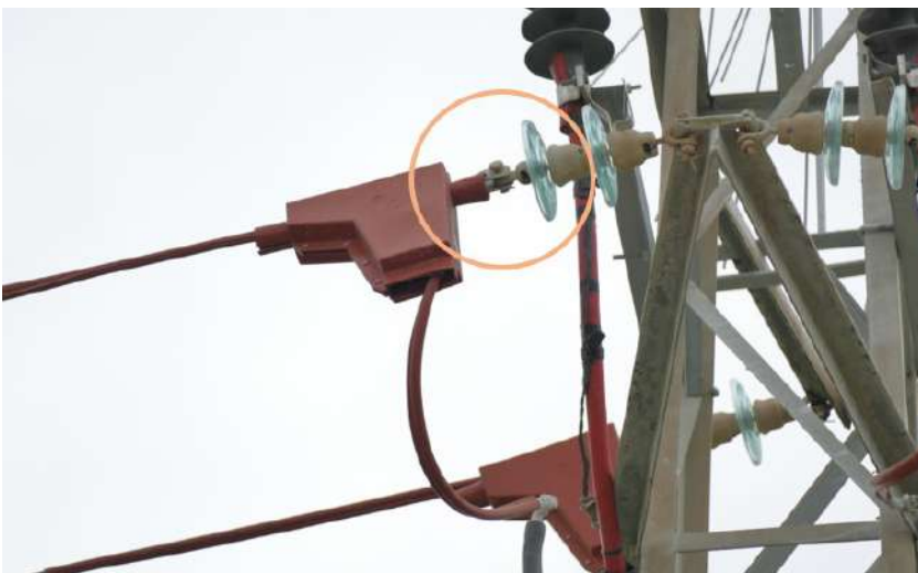
(Top): Disconnected insulation sheath results from suboptimal fitting, highlighting the importance of precise installation for effective bird protection (Bottom): The insulation inadequately shields the entire live metal component, potentially compromising safety
