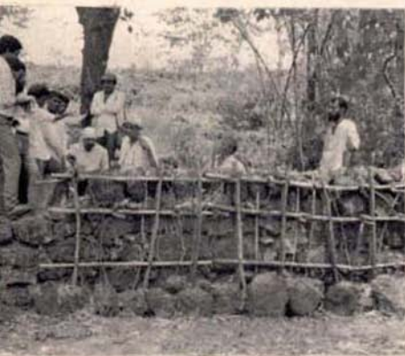
Small crib dam in Ratnagiri district, Maharashtra, built cheaply with local labour.
